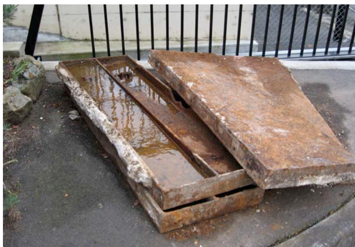
Rusted targets prior to restoration
